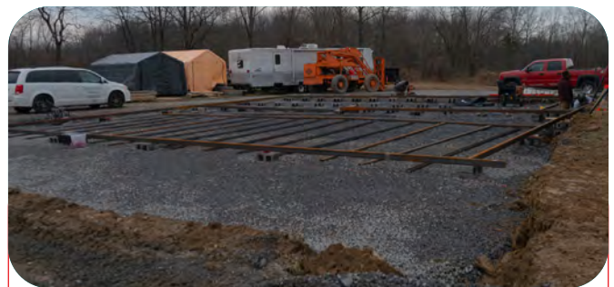
Our outdoor mockup slab capable of supporting two-story mockups up to 50 feet long.
